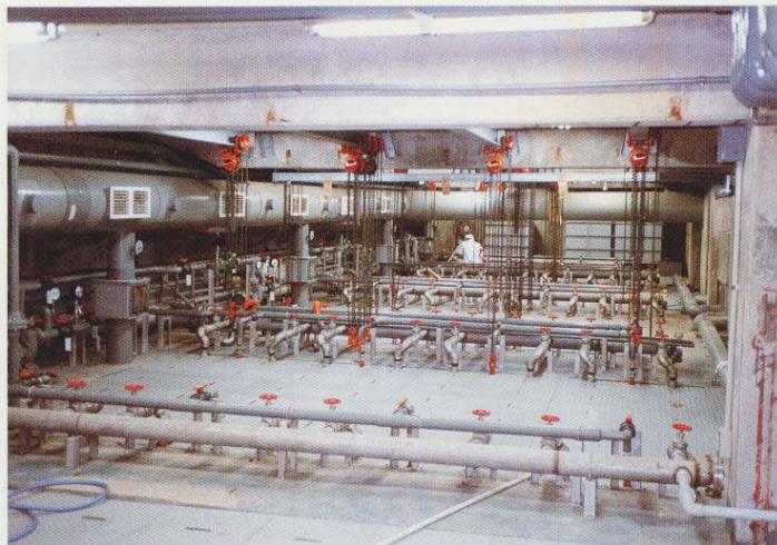
General view of system
