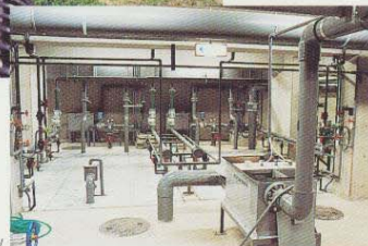
Water treatment facility
